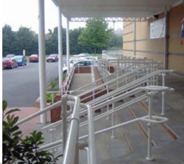
Right: ADA Compliant Railing for Public Access
